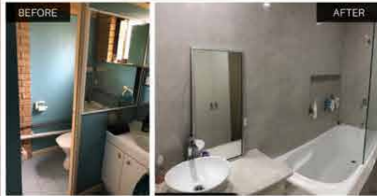
This brand new bathroom on the ground floor of the Chaplain's Residence is a welcome addition to the home—and isn't it pretty?!
