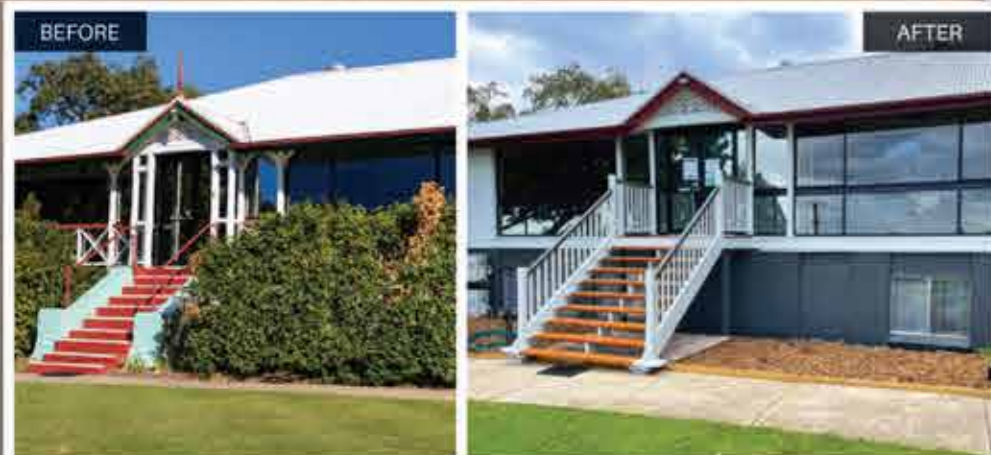
At long last, thanks to your generous giving over several years, we were able to paint the main administration building of the college for the first time in decades. One of our own alumni, professional painter Phil Coates, took on the job single-handedly with more attention to detail and care than we could have hoped for, and the result is outstanding. We were also able to replace the old cement stairs with this beautiful new timber staircase—a place for students to sit and chat between classes and make memories that last a lifetime.
